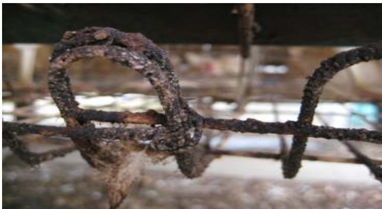
Extent of corrosion is clearly visible after only three months of deployment. The method of using metal primer paint proves ineffective in addressing corrosion in a poultry environment.
