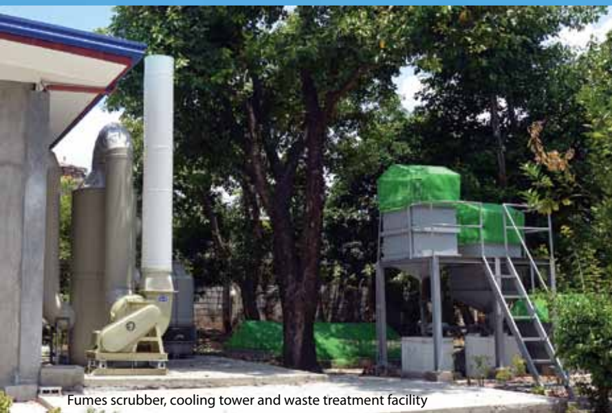
De-ionizing water facility
