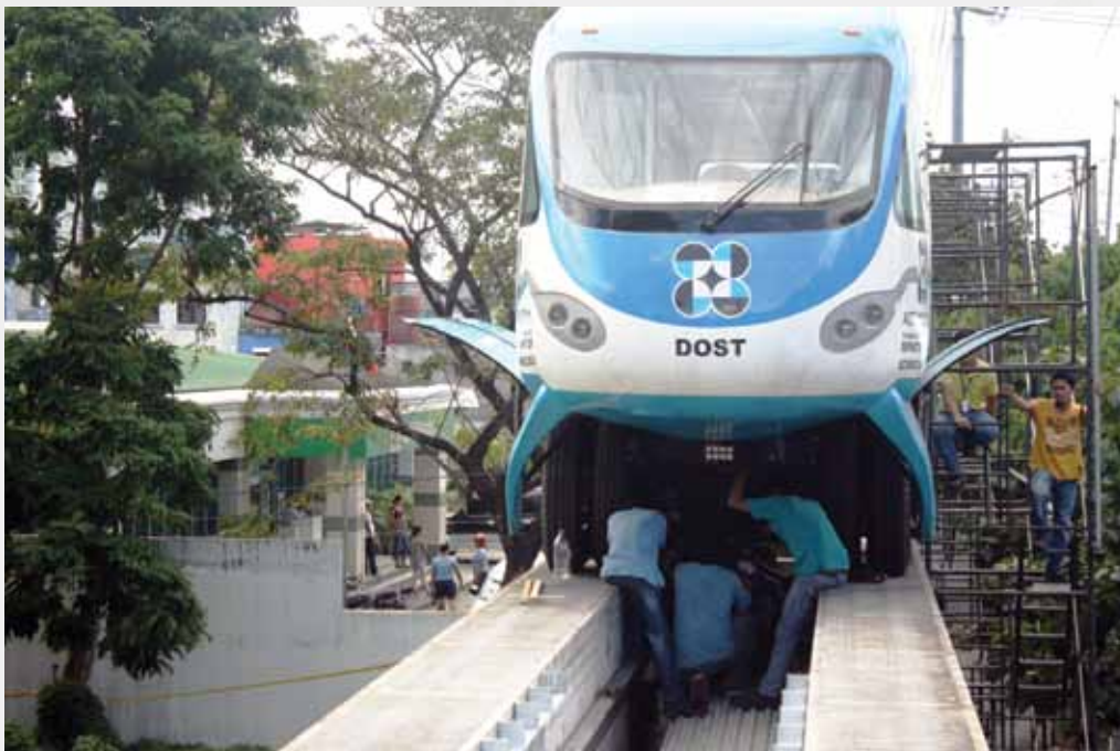
AGT120 staff installing the retainer assembly to bolster the safety design features of the AGT system.
