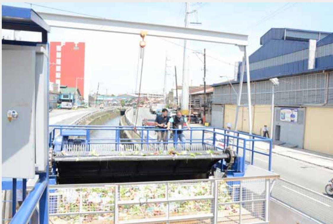
The Automatic Trash Rake facility at Balingasa Creek in Quezon City.
