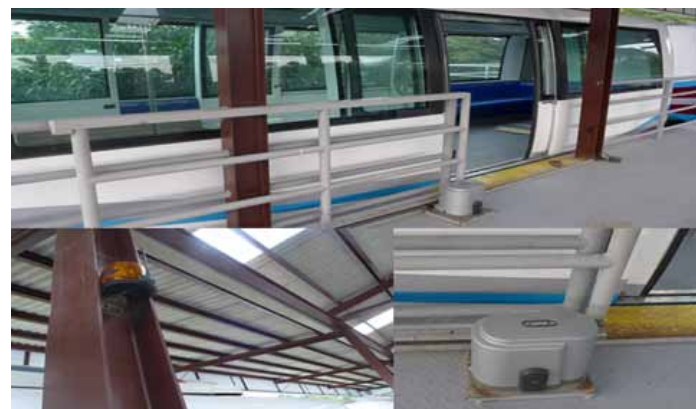
Automated sliding gate at the platform area of the station equipped with motor, flashing light and safety sensor.
