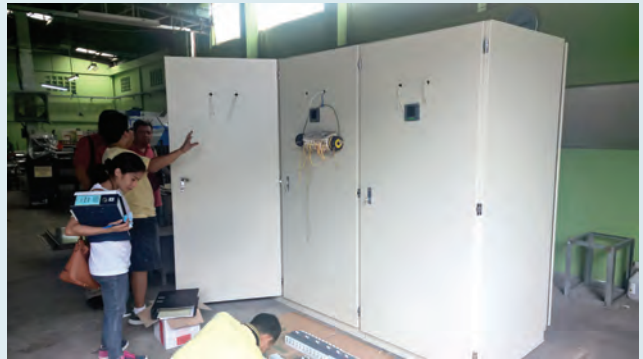
Electrical control panel board
