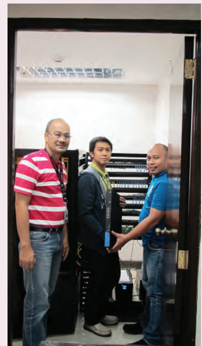
PMD-MIS connecting all work stations to the MIRDC LAN.
