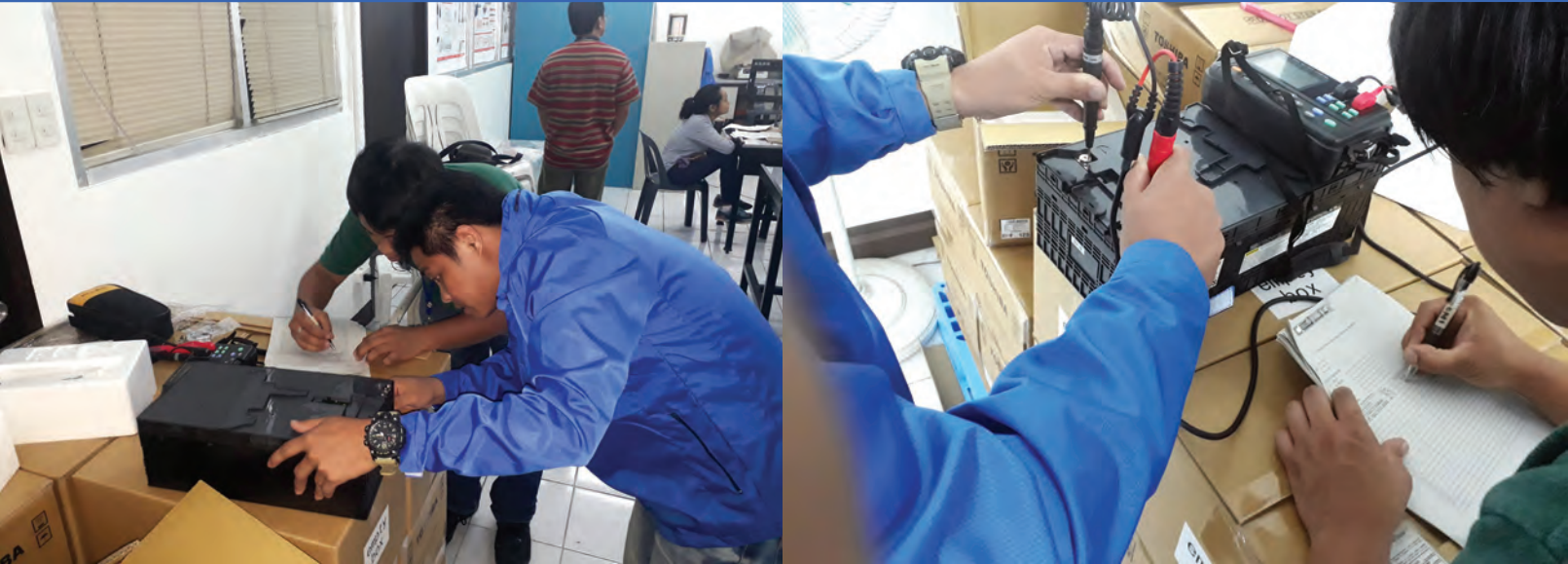
Road Train project staff check and test the newly arrived lithium titanium oxide (LTO) batteries that will be installed in the Light Hybrid Electric Road Train
