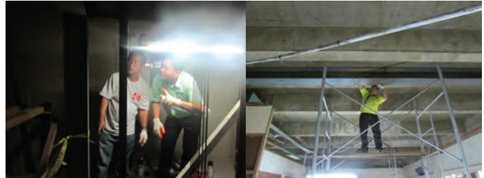
NDT staff perform testing at the ongoing construction of elevator and retrofitting of MIRDC Gold Building
