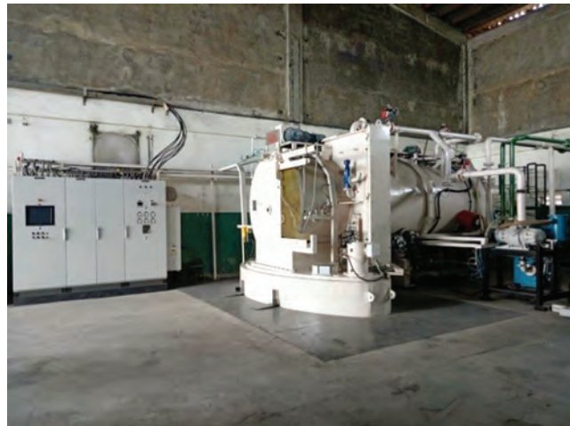
The newly installed Vacuum Carburizing Heat Treatment Facility installed at the MIRDC Surface Engineering Bldg.
