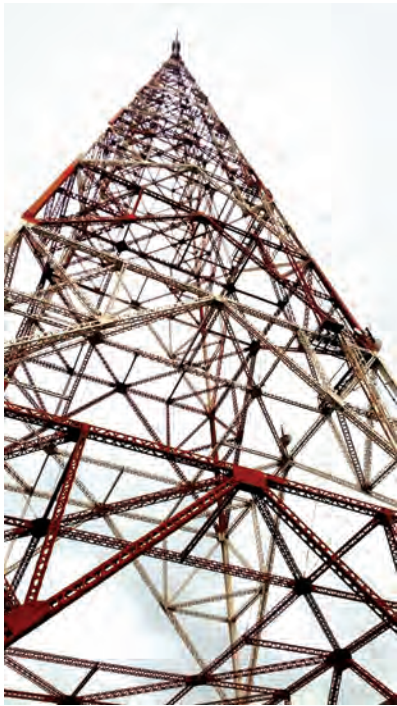
IBC Transmission Tower which underwent non-destructive test using pXRF
