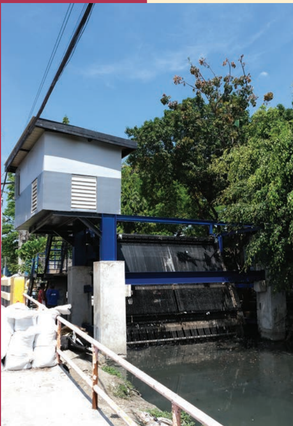
The installed Automatic Trash Rake which will improve the flood control operations in Malabon.
