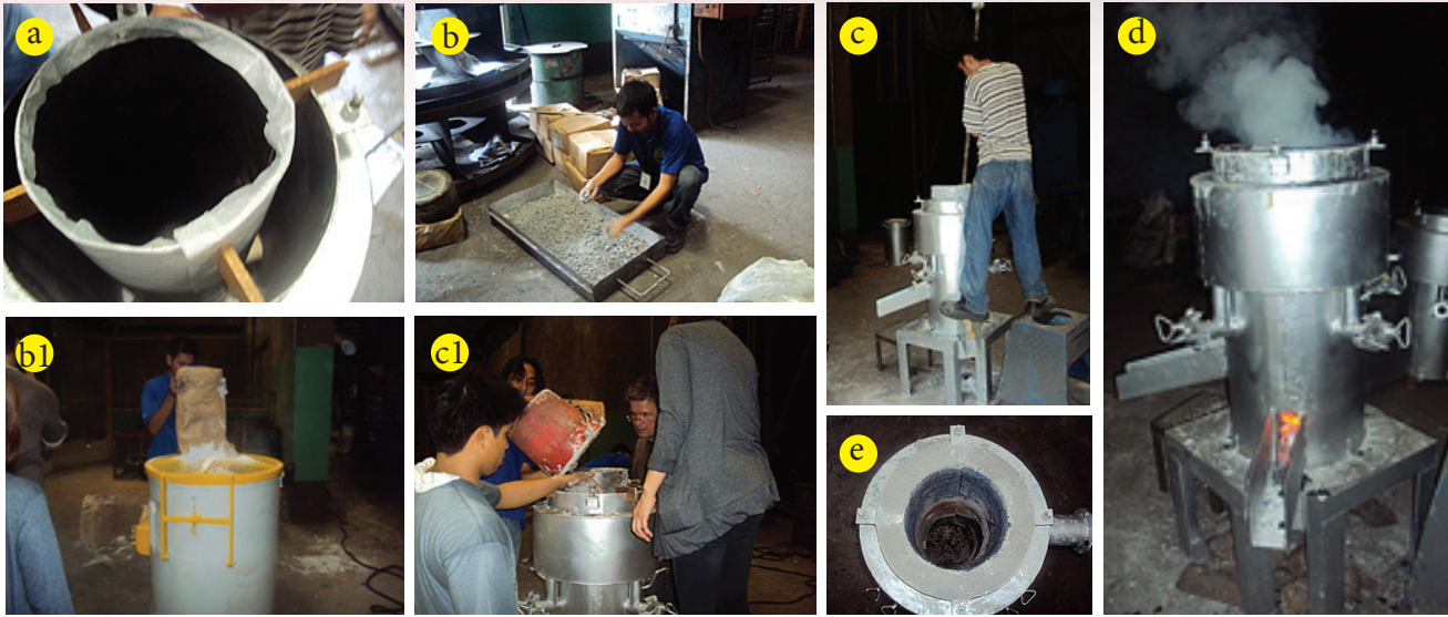
Fig. 3: (a) Preparation of the furnace shell for lining; (b) Preparation of the phosphate-bonded rammable alumina castable; (b1) Preparation of the hydraulic-chemical free-flow alumina castable; (c) Installation of the rammable lining; (c1) Installation of the free-flow lining; (d) Initial sintering of the lining; (e) Cupola furnace with refractory lining installed ready for full sintering.
