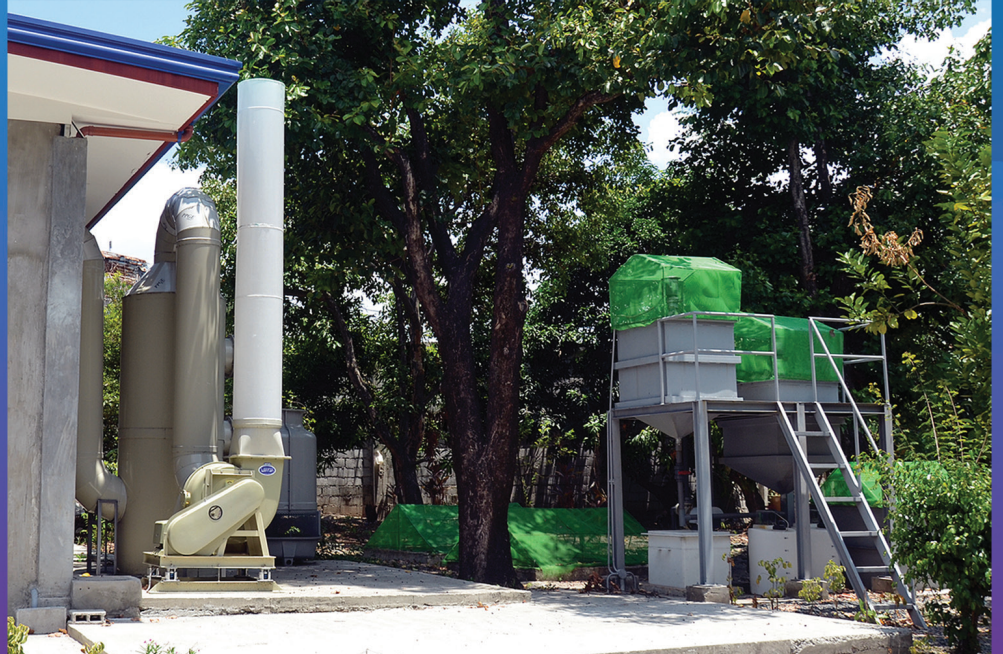
Fumes scrubber, cooling tower, and waste treatment facility
