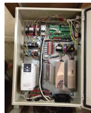
Fig. 10. Control panel box
