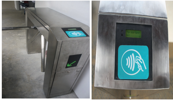
Figure 2. Automatic Turnstile Gate (L) Entry Gate, (R) Card Reader
