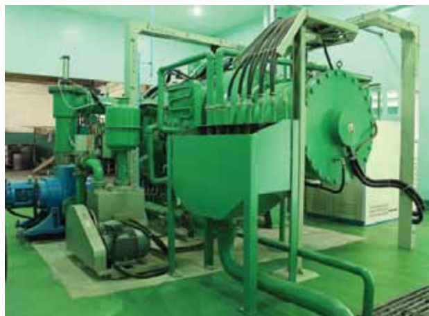
Figure 8. The Water Collection Tank
