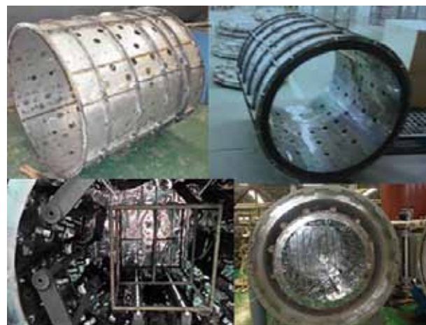
Figure 2. The picture shows (clockwise) the fabrication of the heating chamber. It started with the rolling of the sheet metal and structural reinforcement. The chamber is then insulated. At the lower right, the tubes for evacuation are welded and the whole heating chamber is placed in the outer shell vessel. At the lower left, shows the graphite heaters are configured.
