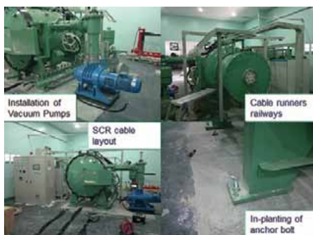
Figure 6. Images above show the integration of the systems as part of the commissioning and training activities
