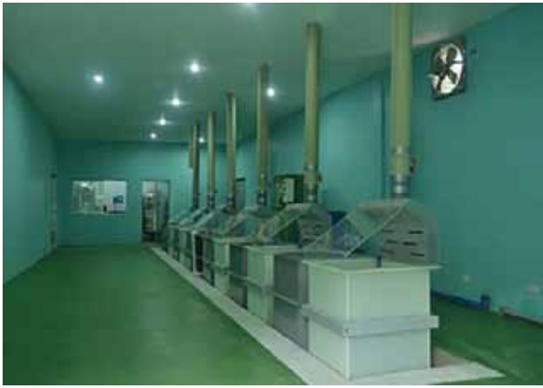
Figure 1. The anodizing line (tanks, rectifiers, and chiller)
