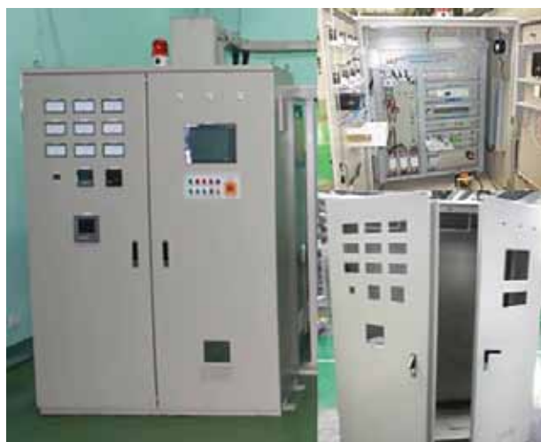
Figure 5. The images presented show the development and installation of Instrumentation on the control panel cabinet
