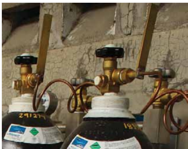
Figure 7. Cylinder and pigtail connection. The arrows below show the connection of pigtail from the nitrogen cylinder (source) to the main pipeline orifice. Leak is most likely to occur at these points if improperly set or connected.
