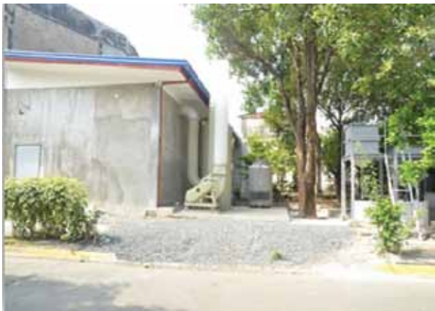
Figure 3. Fumes scrubber, cooling tower, and waste treatment facility
