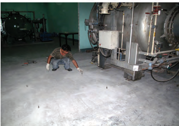
Figure 2. Civil works of the flooring which will serve as permanent location of furnace at Heat Treatment Facility.
