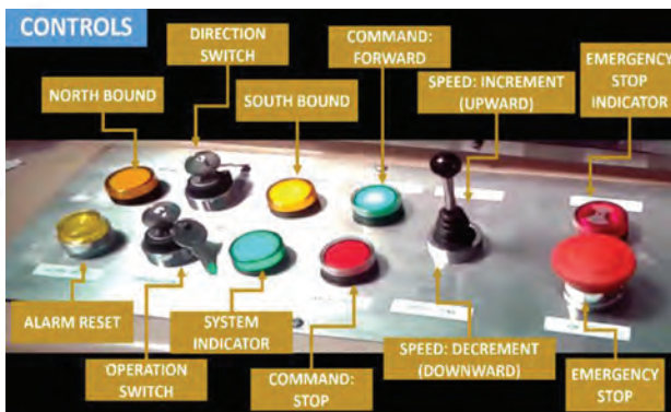
Figure 7. Control panel board
