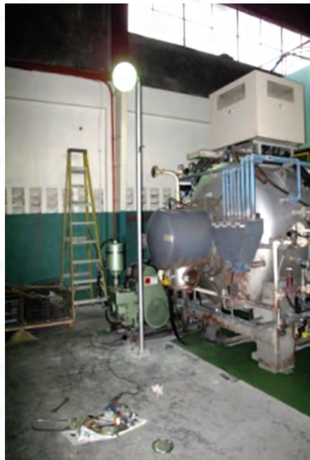
Figure 3. Installation of nitrogen line to the furnace for quenching of heat treated metals.
