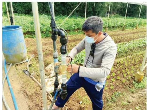
Figure 4. Assembly of Solenoid Valve Bypass to each sprinkler line
