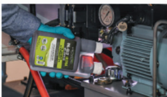
ADD/INJECT FLOURESCENT DYE INTO SYSTEM
