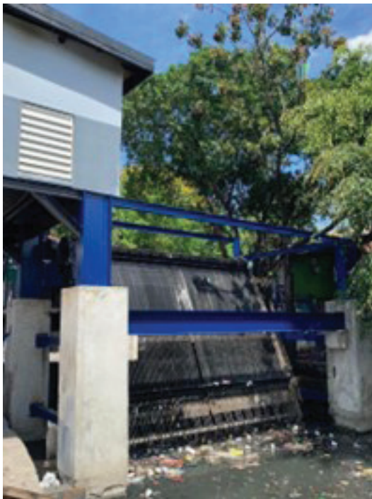
Fig. 4. Automatic Trash Rake Facility
