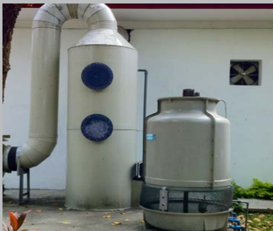
Scrubber controls air pollution and cooling tower transfers process waste heat to the atmosphere.
