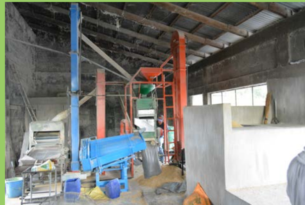
Retrofitted Compact Rice Mill System in CAMPC, Science City of Muñoz, Nueva Ecija.
