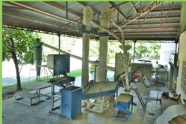
Retrofitted Compact Rice Mill System in PHiMech Science City of Muñoz, Nueva Ecija.
