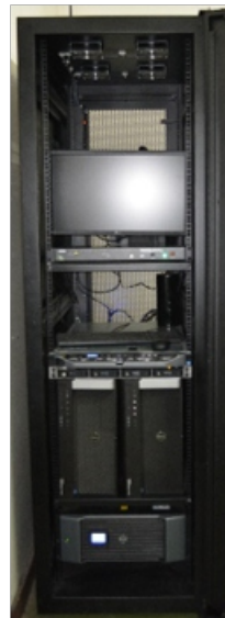
64 core - FEA Supercomputer
