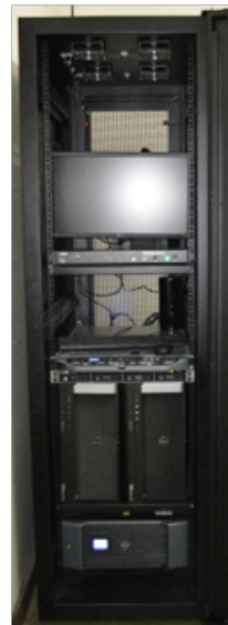
64 core - FEA Supercomputer
